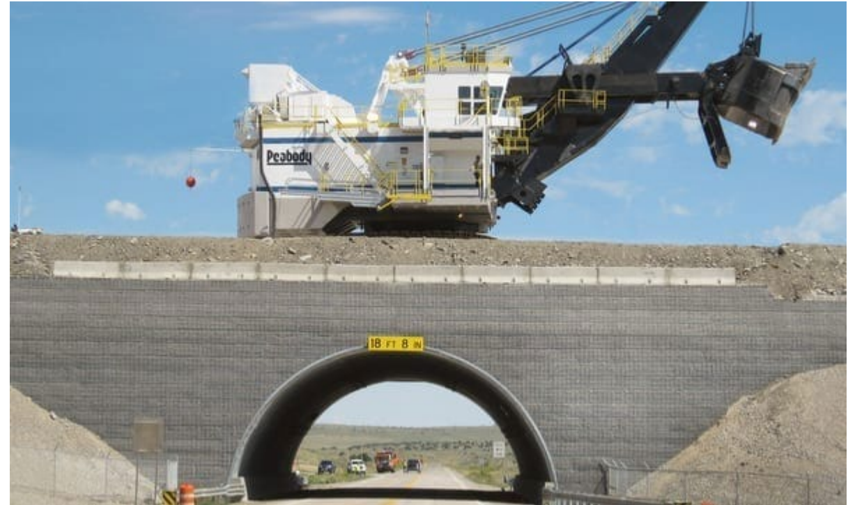
Power shovel moving across NM 509 at the El Segundo/Lee Ranch mine. From ailmining.com.
