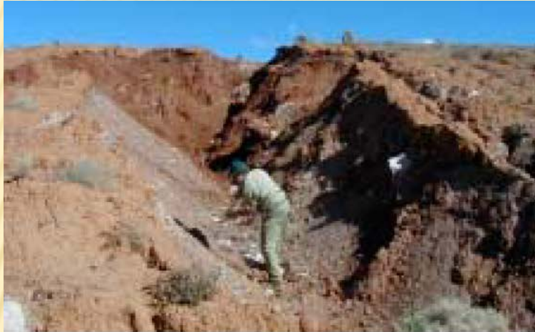
Tunnel collapsed to form a gully
