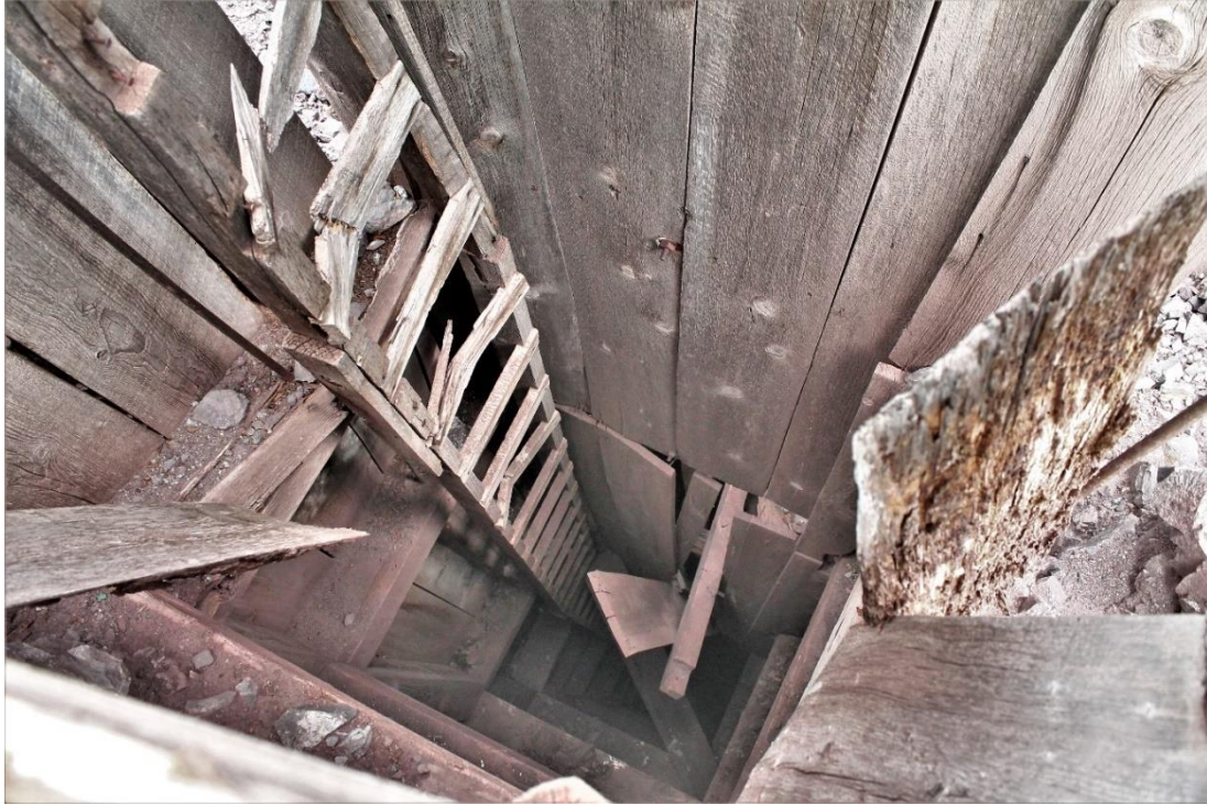
Figure 13. Mag4-S1 (NMSO0377); interior of shaft. Note the broken rungs on ladder and other indicators of instability. This shaft is >300 ft deep.
