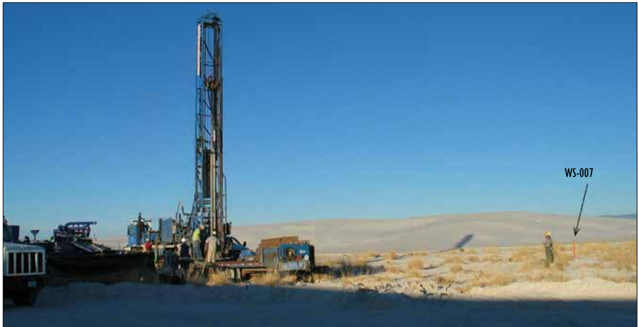
Figure D1. Photo of drilling site for pumping test wells, WHSA. WS-007 is a preexisting shallow monitoring well at the site.
