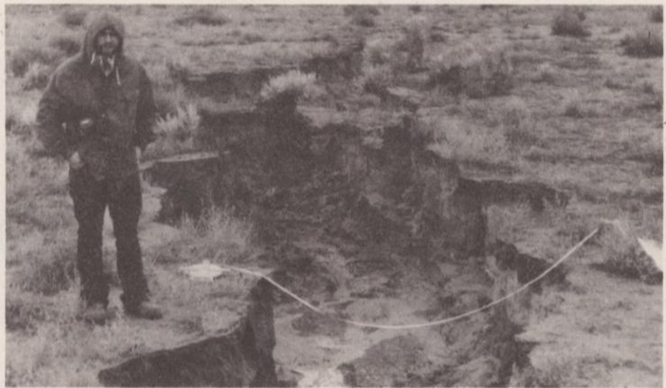
Figure 3—A second view of the same fissure, but in this case looking north from the same vantage point as above. Surface runoff during heavy rainstorms flowed into a portion of the initial crack to produce the fully-developed fissure shown here.
