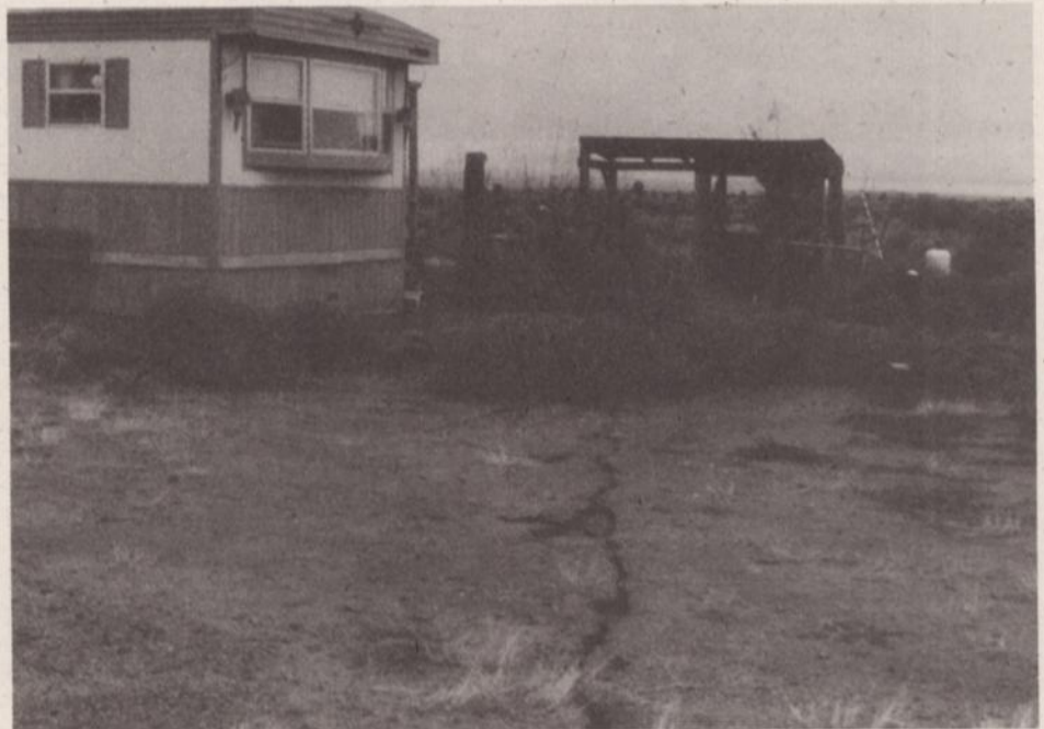
Figure 2—An incipient earth fissure in the Mimbres Basin, which first appeared in 1984. View is toward the south. Total length of the crack in 1984 was 454 m (1480 feet). This portion of the crack had not yet been widened by erosion when the photo was taken. Earth fissures have been documented at 13 separate locations throughout the Mimbres Basin (Contaldo, 1989).
