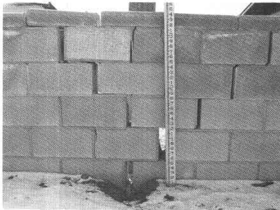
FIGURE 4—Concrete-block wall that was cemented flush originally. The hole in the ground is called a sótano , which literally means basement or cellar but, in this case, signifies an unexplained hole that, if found in a field, could drain much of the surface water directly to the subsurface.
