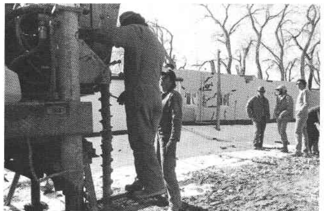
FIGURE 9—Drilling operation in front of a house whose owners have patched the numerous cracks that developed while they were on vacation in the summer of 1984.
