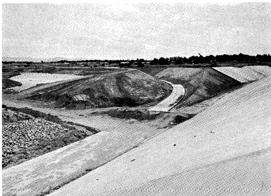
INTERSECTION OF EMBUDO DRAIN AND EMBUDO ARROYO With the North Diversion Channel, seen at Menaul Boulevard bridge over the channel.
