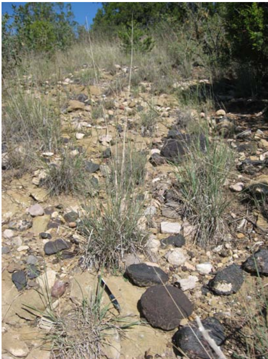
35. Iron-rich lag placer deposits are common within and below eroded Qm deposits on Santa Rosa Sandstone. New UTM 456600, 3715800. Pencil is about 15 cm long.
