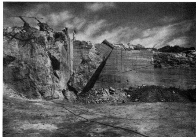
FIGURE 13—After cutting, large travertine slabs are tipped over, onto cushioning debris, using hydraulic wedges before processing into blocks or rubble.
