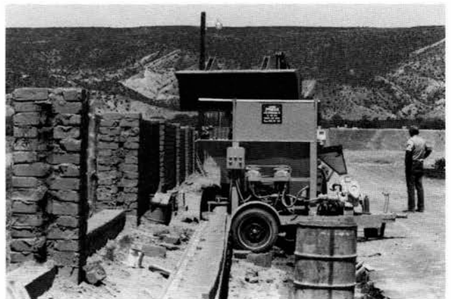
FIGURE 4—Earth Press III pressed-earth-block machine set up near wall under construction. Coyote Adobe Inc. building site, Velarde, New Mexico.
