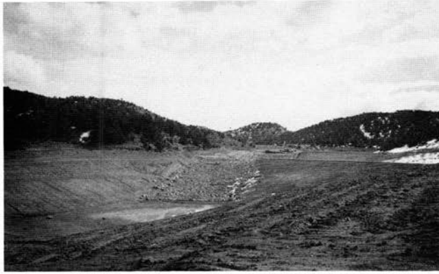
FIGURE 9—Spillway lined with clinker at Peabody Black Mesa mine. Material is taken directly from a borrow pit nearby; the size of the aggregate is variable.
