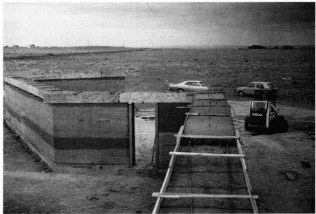
FIGURE 6—Thick rammed-earth walls after forms have been removed at Huston home near Edgewood, New Mexico, with a freshly poured concrete bond beam. Note tamped soil layers with different amounts of water. When completely dry, the walls will be nearly the same color, but layers will remain variable due to differences in grain size. After stucco is applied, the walls will appear monolithic.
