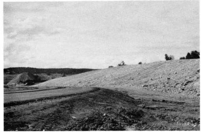
FIGURE 10—Rock “mulch” used to stabilize slope along temporary road. Road also has base of clinker.
