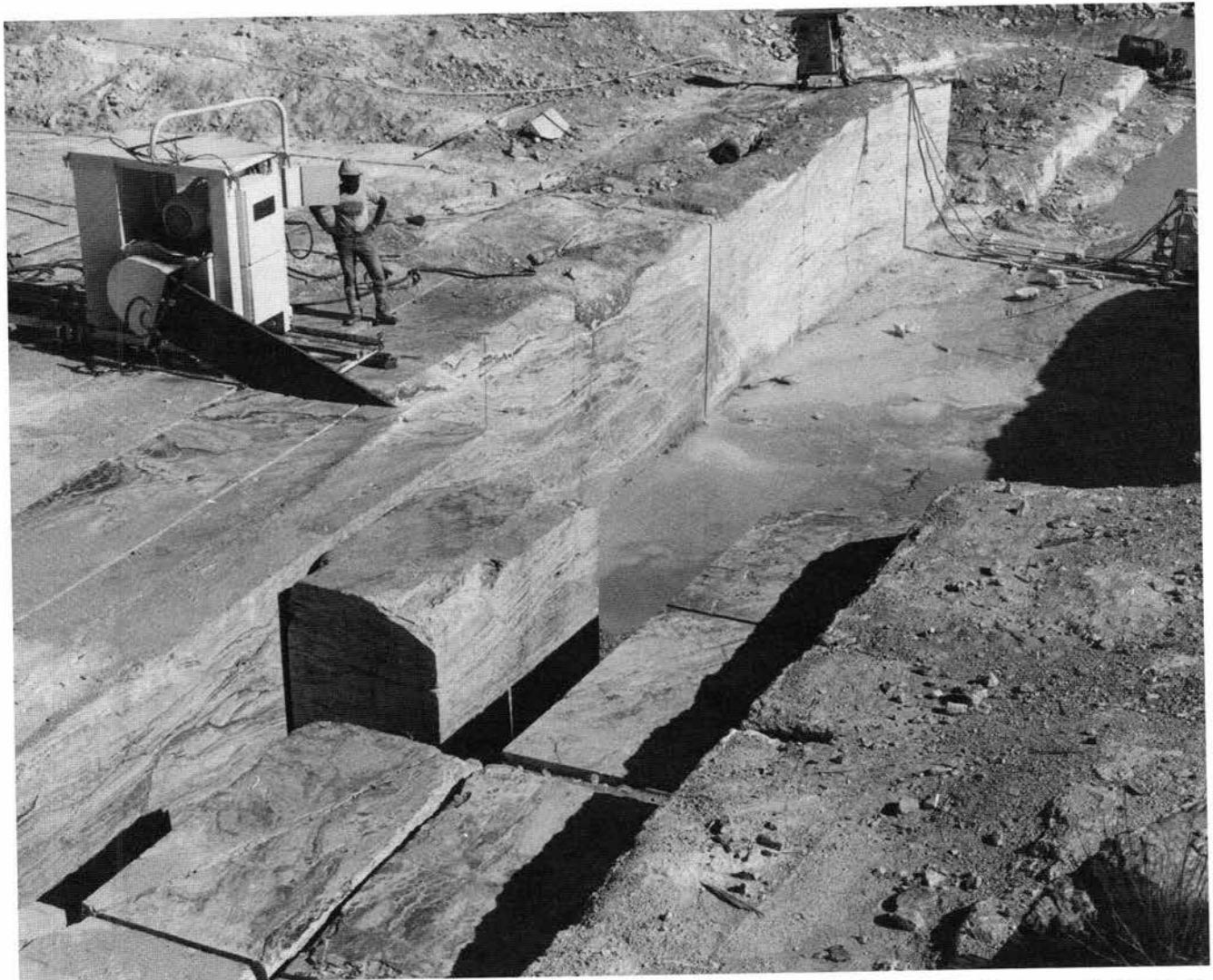
FIGURE 10—New Mexico Travertine quarry west of Belen, New Mexico, in Scheherazade travertine (trade name). Diamond-impregnated belt saw is cutting 1 \frac{1}{2} inch channel up to 10 ft deep. Wire saw at upper right is "pulling floor" on a block previously cut by the belt saw.
