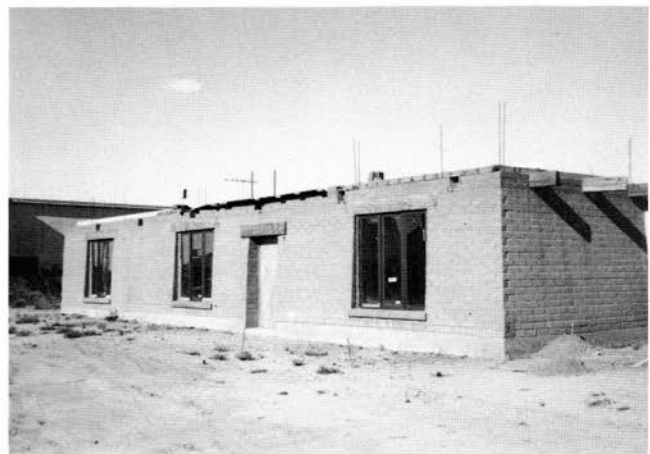
FIGURE 76—W. S. Carson CINVA-Ram pressed-earth-block house under construction in 1980 near Columbus. Note vertical steel reinforcements.
