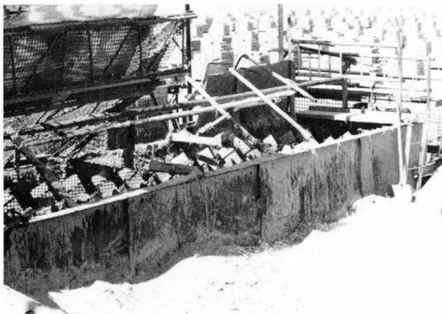
FIGURE 62—Close-up of the large 4 x 6-ft pugmill. Adobe Factory adobe yard, Alcalde.
