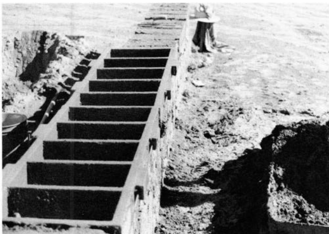
FIGURE 55—Two five-mold wooden forms set on corral wall under construction and ready for filling. Adobe Corrals Project, Corrections Industries, Santa Fe.
