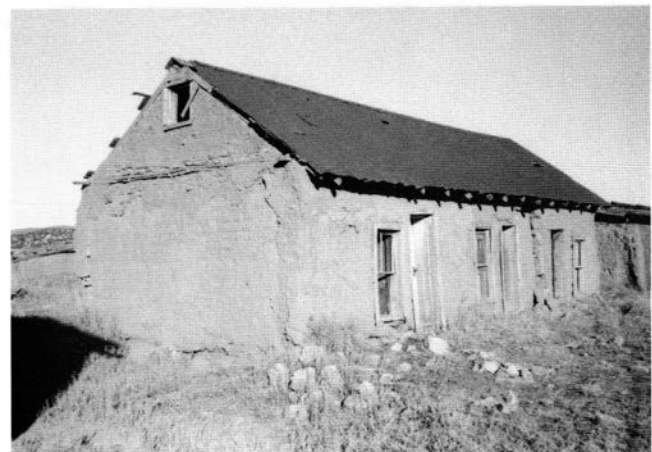
FIGURE 28—Old adobe home, San Jose. The owner has added a corrugated iron roof to protect the adobe structure.
