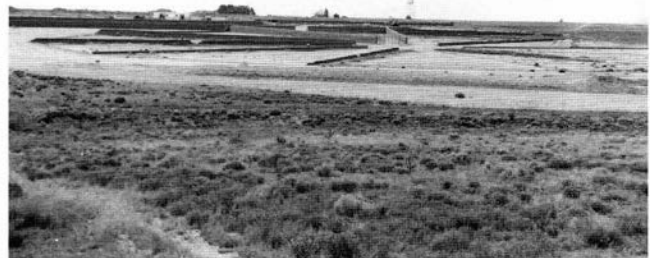
FIGURE 53—View of the wild-horse corrals under construction during the summer of 1988. The walls are 7 ft high, 261 ft long, and 16 inches thick. Adobe Corrals Project, Corrections Industries, Santa Fe.
