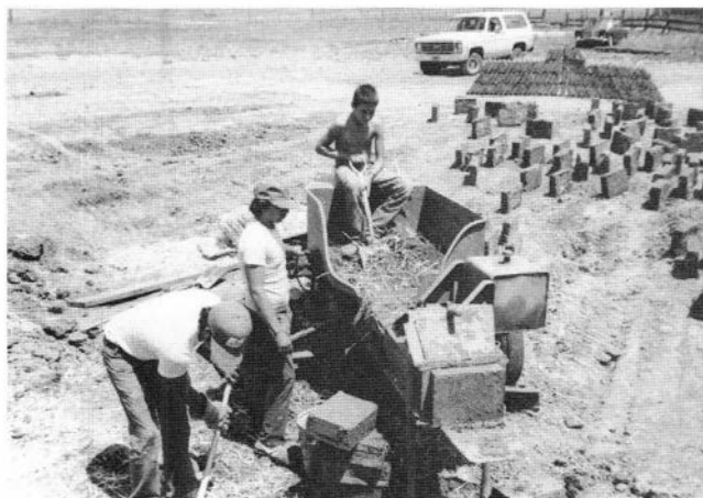
FIGURE 70—Porta Press in operation during the summer of 1980. David Griego building site, Ledoux.
