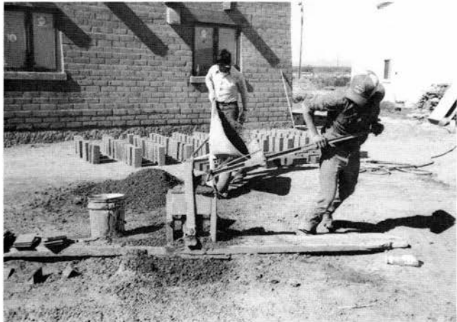
FIGURE 74—Applying pressure to the soil mixture to produce the pressed-earth block from the CINVA-Ram. W. S. Carson building site near Columbus.
