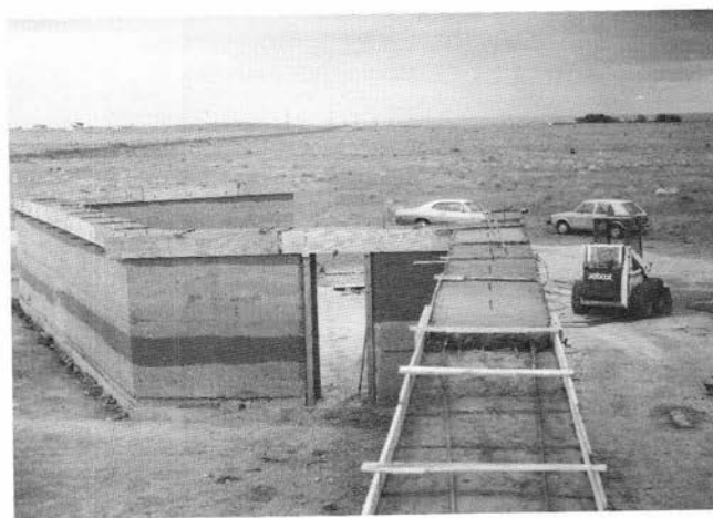
FIGURE 97—Rammed-earth walls and pouring of the concrete bond beam. Note the soil colors and the layering produced by tamping. Huston Construction Company building site, Edgewood.
