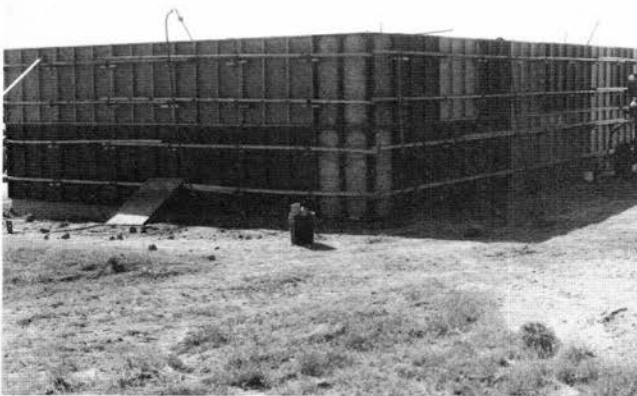
FIGURE 93—Setting of the wooden forms for construction of the rammed-earth walls, Huston Construction Company building site, Edgewood.
