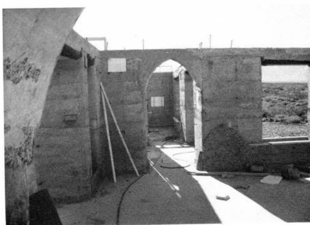
FIGURE 99—Rammed earth walls with arches and windows. Note concrete bond beam and form for concrete window sill at lower right. Soledad Canyon Earth Builders building site, Mesilla.
