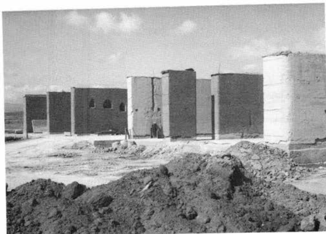
FIGURE 96—Huston house under construction, Edgewood. Note thickness of exterior walls (36 inches) and interior wall (16 inches) after removal of wooden forms.
