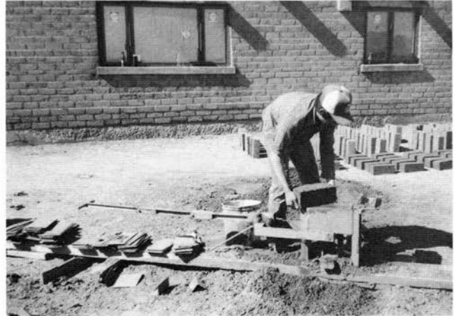
FIGURE 75—Removing the pressed-earth block from the CINVA-Ram mold. The pressed-earth block is then placed in the yard to dry. W. S. Carson building site near Columbus.
