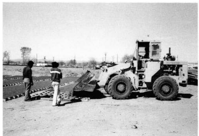
FIGURE 51—Front-end loader dumping the adobe mud into the ladder molding forms. New Mexico Earth adobe yard, Alameda.
