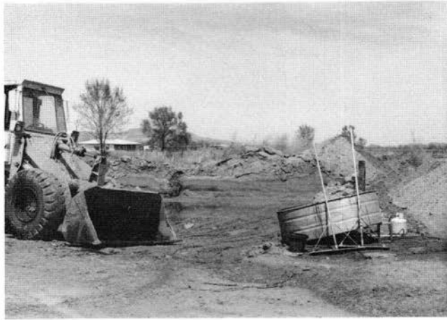
FIGURE 29—Mudpit at the Rio Abajo Adobe Works adobe yard, Belen. Asphalt emulsion from tank on the right and water are added to soil in the center. Mixing is done by the front-end loader.
