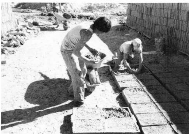
FIGURE 46—Packing the adobe mud into a four-mold wooden form. Eloy Montano Sand & Gravel adobe yard, Santa Fe.
