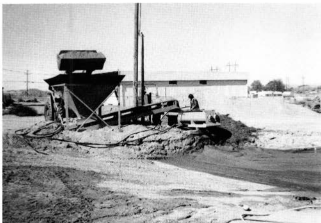
FIGURE 49—Front-end loader placing soil mixture into pugmill, where the adobe mud is mixed and then dumped into the mudpit by the conveyer system. New Mexico Earth adobe yard, Alameda
