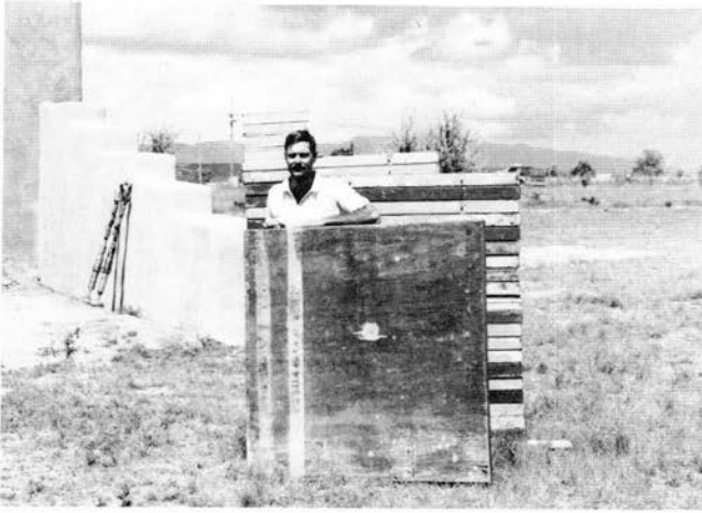
FIGURE 92—Stan Huston displaying the 4 × 4-ft wooden forms used in rammed-earth construction. Huston Construction Company building site, Edgewood.
