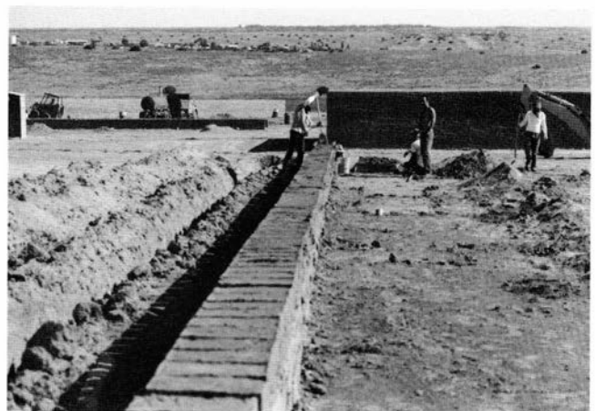
FIGURE 56—Packing adobe mud into the five-mold wooden forms to produce bricks directly on the wall. Adobe Corrals Project, Corrections Industries, Santa Fe.
