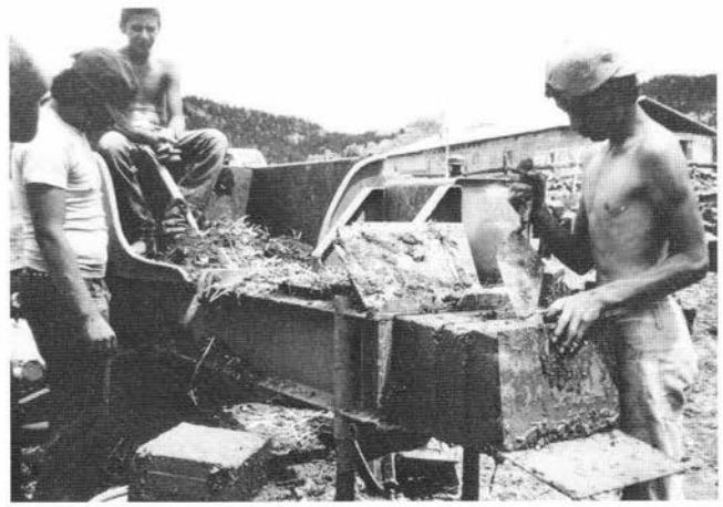
FIGURE 71—Cleaning Porta Press pressed-earth blocks prior to stacking in the yard to dry. David Griego building site, Ledoux.
