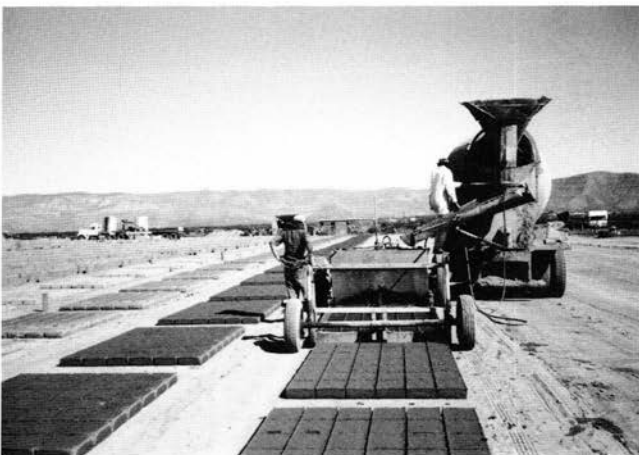
FIGURE 66—The ready-mix truck dumping the mixed adobe mud into the hopper of the adobe layer, which produces 42 standard-size adobe bricks per laydown. The Adobe Patch adobe yard, La Luz.
