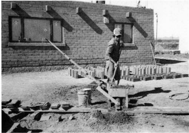
FIGURE 73—Loading the CINVA-Ram mold. Note drying pressed-earth blocks near building. W. S. Carson building site near Columbus.
