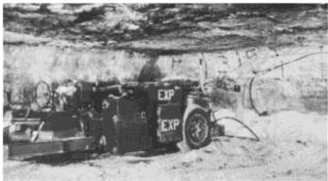
FIGURE 4—AMMONIUM NITRATE AND FUEL OIL (AN/FO) IS BLOWN INTO THE DRILL HOLES AS THE TUBE IS WITHDRAWN.
