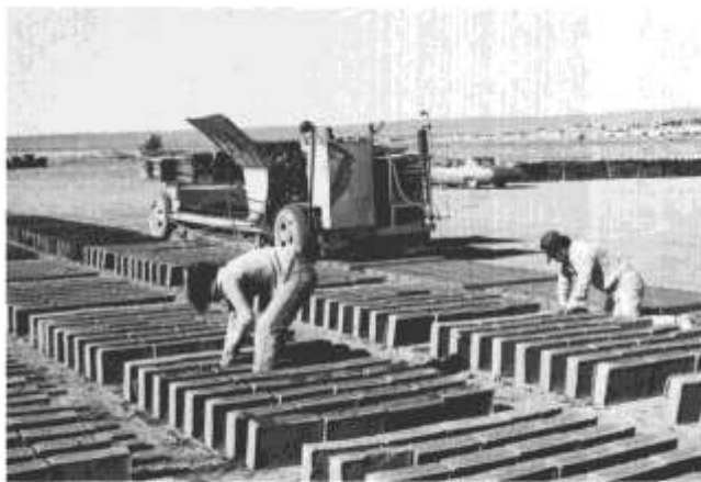
FIGURE 15—SELF-PROPELLED ADOBE LAYER AWAITING A LOAD OF MUD DELIVERED FROM THE MUDPIT BY THE FRONT-END LOADER. Note adoberos turning and cleaning the adobes at the Western Adobe yard in Albuquerque.
