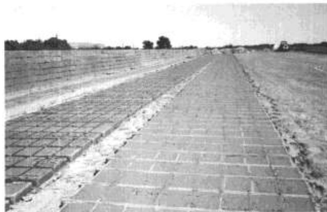
FIGURE 9—ADOBES DRYING IN WOODEN FORMS AT THE RIO ABAJO WORKS AFTER THE MUD HAS BEEN POURED AND RAKED SMOOTH. FORMS will be removed the same day after the mud has partially dried and shrunk from the mold sides.
