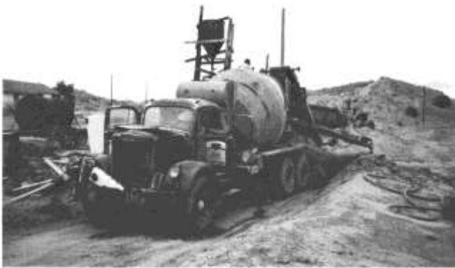
FIGURE 11—A 7.5-YD 3 READY-MIX TRUCK MIXES THE ADOBE SOIL, WATER, AND ASPHALT EMULSION AND DELIVERS THE MIXTURE TO WOODEN FORMS FOR POURING. Photograph taken at the Adobe Farms yard in Española.
