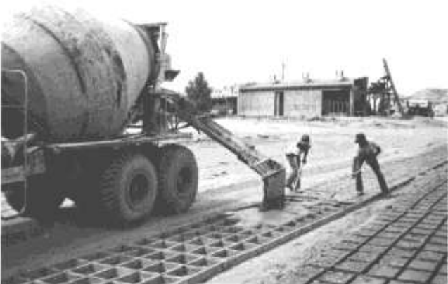
FIGURE 12—POURING, RAKING AND LEVELING OF ADOBE MUD IN WOODEN FORMS AT THE ADOBE FARMS YARD IN ESPAÑOLA.
