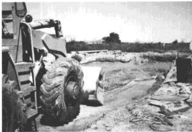
FIGURE 8—A MICHIGAN MODEL 75-3 FRONT-END LOADER WITH A 2-YD 3 BUCKET WORKING A CEMENT-LINED MUDPIT AT THE RIO ABAJO ADOBE WORKS IN BELEN.
