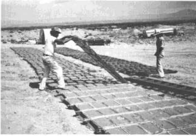
FIGURE 10—AFTER THE ADOBE MUD HAS PARTIALLY DRIED, WOODEN FORMS ARE LIFTED AND RELOCATED FOR THE NEXT MUD POURING. Photograph taken at the Adobe Enterprise yard in Albuquerque.
