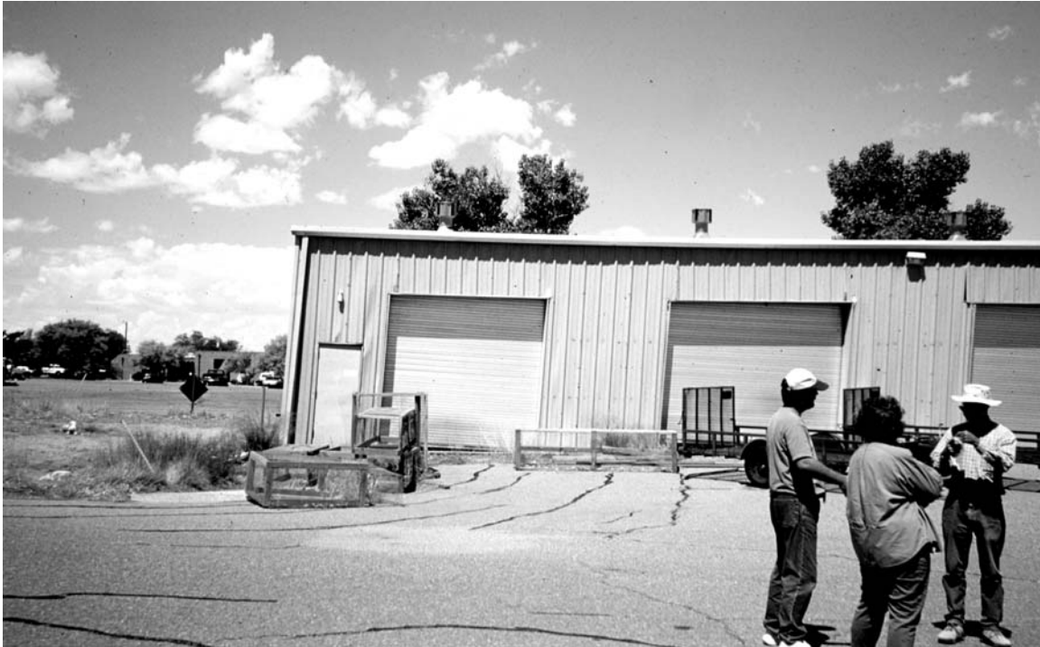
Figure 2-14. Photograph of the south end of the Kaibab Warehouse #1 facility at Montessa Park. Note the arcuate cracks in the asphalt, which have been repaired. These cracks encircle the exposed soil to the left of the building. The doors of this warehouse are out of plumb and rest on the foundation along the right side, but are not supported to the left. Dave Love is at right side of photograph.
