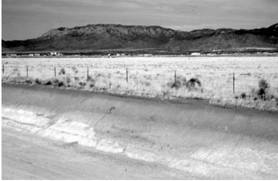
Figure 2-13. Recently constructed flood detention pit on east side of Journal Pavilion parking lot. The Sunport soil is about 1.5 m thick and exhibits Stage III+ carbonate morphology. The top of the soil is irregular and has been modified by relatively deep pipes developed into the profile.
