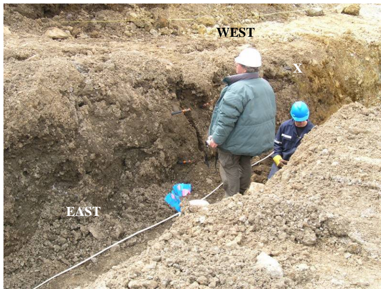
FIGURE A9-54. GHN-LFG-008-H019. Bench 20, south wall showing tension crack in Unit O. Sample GHN-KMD-0088 was collected at location X.
