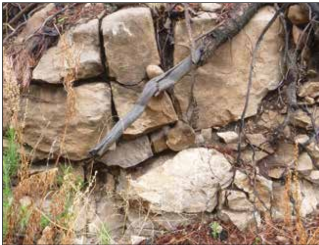
Figure 24. Tree roots penetrate fractured San Andres Formation.
