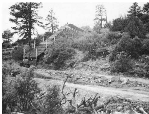
FIGURE 123—Chute, tipple, and storage bin under construction at the Rainbow No. 3 mine. Photo by R. S. Fulton, August 9, 1949.
