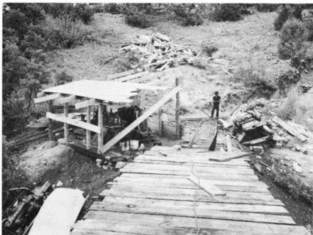
FIGURE 122—Construction at the portal of the Rainbow No. 3 mine. The hoist is under the crude shed. Photo by R. S. Fulton, August 9, 1949.
