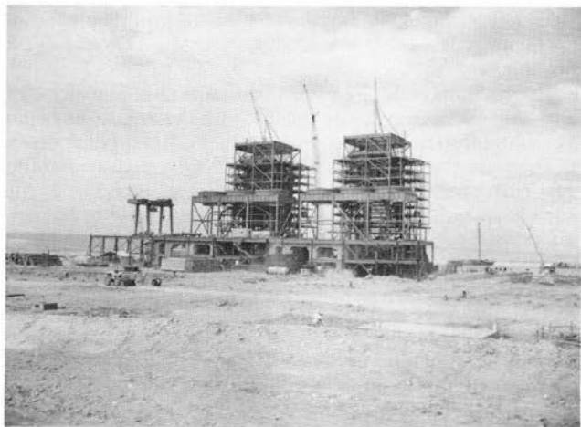
FIGURE 71—View to the north of Arizona Public Service Company plants Nos. 1 and 2 under early construction at the Four Corners powerplant site. Photo by H. B. Nickelson, April or May 1961.
