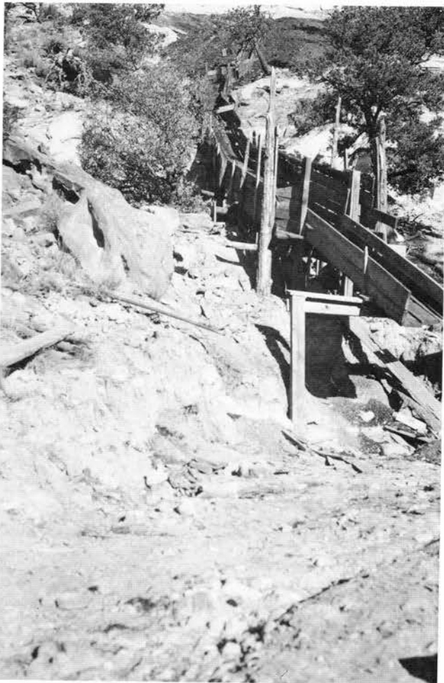
FIGURE 192—Chute built by Mr. Looney on the Looney prospect to transport the coal to the valley floor. Photo by R. D. Reeder, August 19, 1939.
