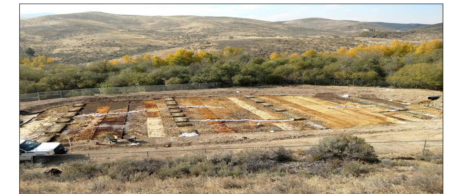
Passive water treatment using cells filled with organic debris to raise pH of water and precipitate metals.
