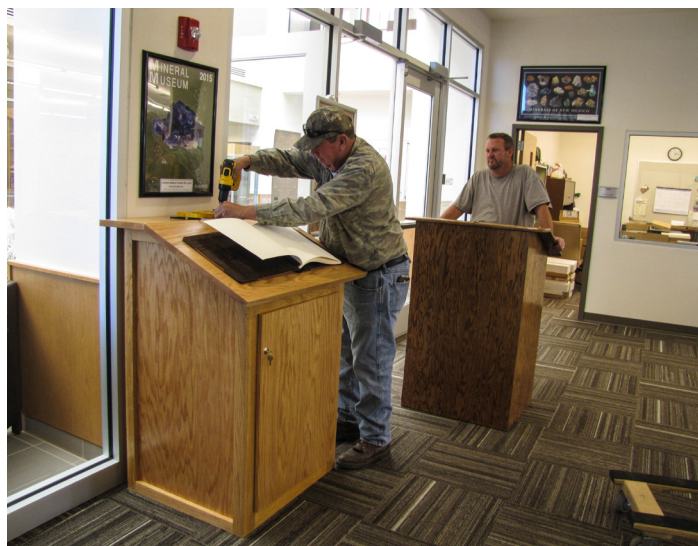
Albert Baca and Brian Wheeler, Bureau carpenter and mechanic (respectively), installing our new guest book pedestal.
