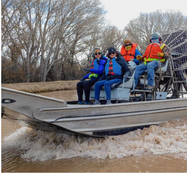
Attendees rode on airboats in the Rio Grande just north of Elephant Butte, where amphibious excavators were dredging sediments in the delta channel.
