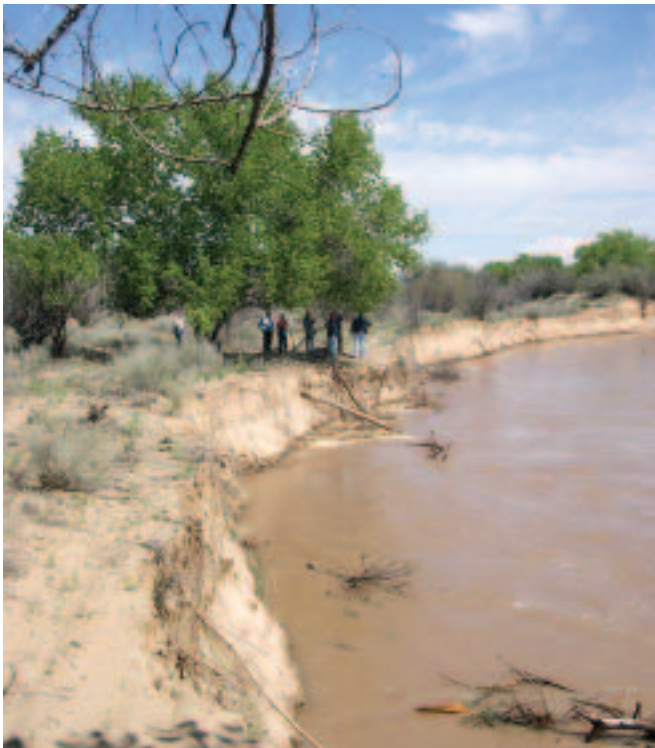
Erosion of river bank at river mile 111, just a few miles below San Acacia, due to high snowmelt runoff in spring 2005. The river is migrating laterally to the left, toward the cut bank.
