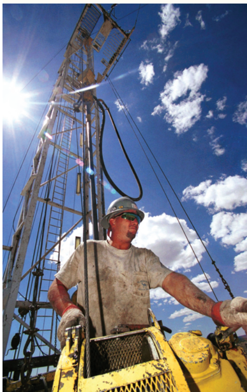
Driller Tom Cumpston on Bearcat Drilling's rig north of Aztec, NM. One of New Mexico's most promising renewable energy resources, the sun, is also visible. Photo by Marc F. Henning.
