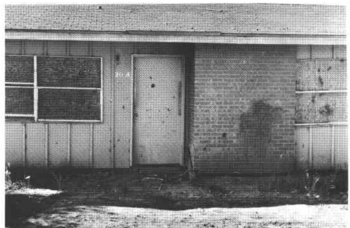
FIGURE 5—Government-subsidized home damaged by subsidence over abandoned coal mines, Sky Village subdivision, Gallup. Photo courtesy of D. W. Love.
