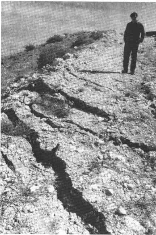
FIGURE 9—Cracks developed in an unimproved dirt road during a September 1991 landslide north of Ft. Sumner, in De Baca County. Approximately 50 cm of rain, well above the average, had fallen during late summer 1991. Highly weathered landslide deposits in the area indicate that landsliding has been common in the past. De Baca County Disaster Preparedness Coordinator Bobby Russ is included for scale.
