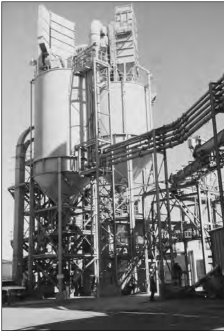
FIGURE 8—Phoenix Cement classifying and storage facility at Cholla Generating Station, Joseph City, Arizona.
