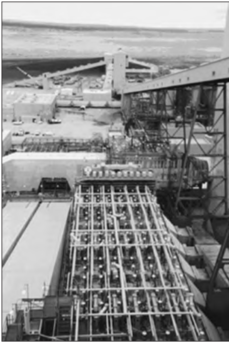
FIGURE 2—Electrostatic precipitators in foreground. Coal stockpile in background and conveyor system on right side of photo. Coronado Generating Station, St. Johns, Arizona.
