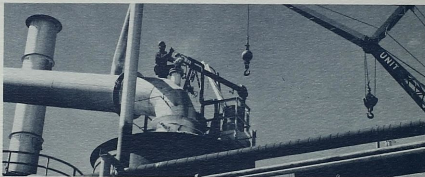
Sulphuric acid from this plant is used to dissolve uranium into solution during processing at Kermac mill—the nation's largest.
